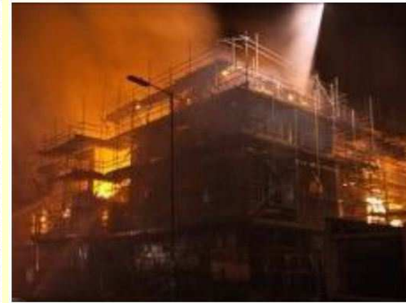
Basingstoke 2010 Timber Frame Arson
